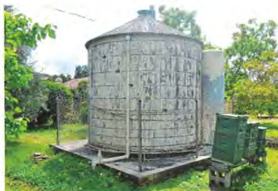
Figure 25. Water Tank at Messina Orchard. Source: Messina Orchard National Register Nomination.
